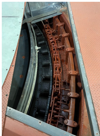
Figure 2. Generator air gaps leave virtually no room for error or lack of precision. Source: Kaman Measuring
